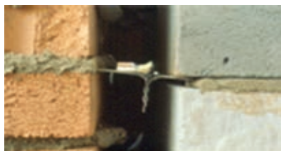
Wall tie incorrectly sloping toward inner leaf.
