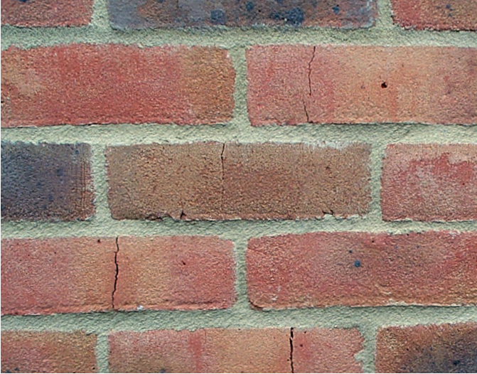
Fire-cracks in clay brick. Cracks do not extend into the mortar joint suggesting their presence when built in.
