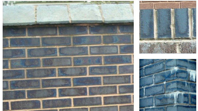
Iridescent appearance caused by light diffraction through fine cementitious material that has leached from mortar
